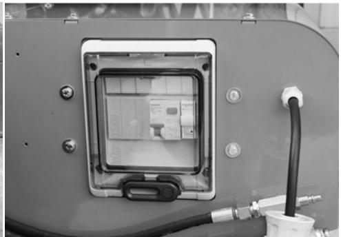
Fig. 89 Main electric switch
