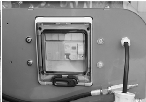
Fig. 158 Main supply switch
