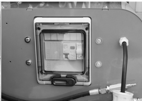
Fig. 160 Main supply switch
