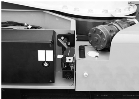
Fig. 133 Battery cut out switch
