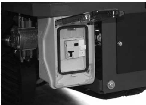
Fig. 85 Main electric switch
